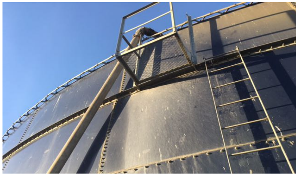
Slurry Tank at Winnifred Colony Dairy Medicine Hat, AB CA. Continuously applied, no sludge build up problems over 21yrs.
